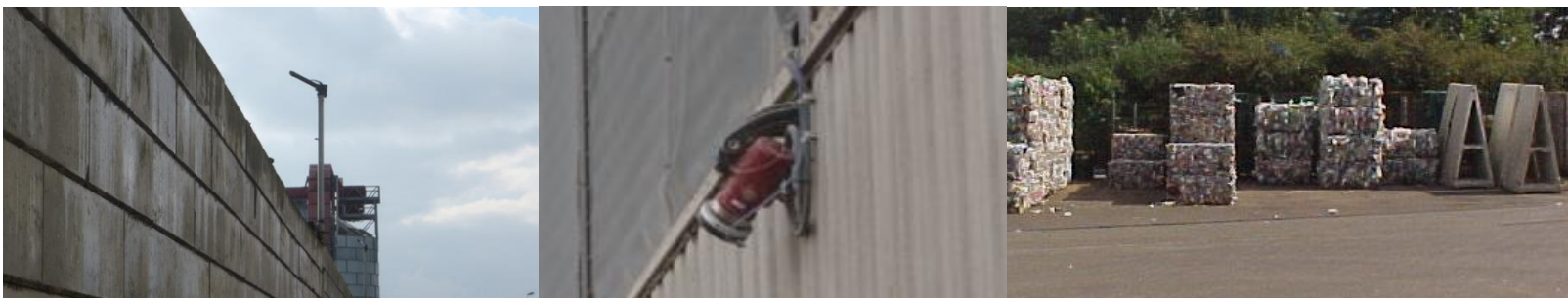
From left: Water deluge head mounted above external waste storage bunker wall (example only – deluge etc systems can be mounted lower or direct on walls), camera-type detector in external use above a waste bunker, standard bale storage ('A' frames in place for use as fire walls as required)
