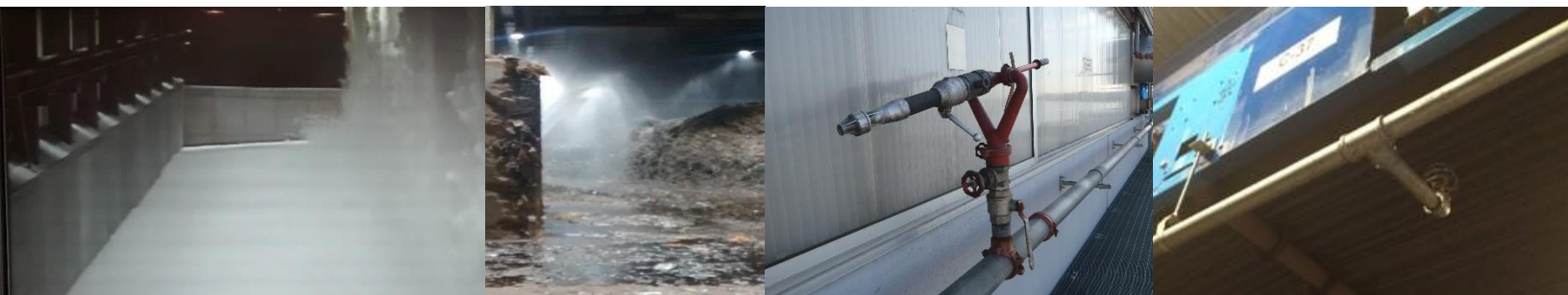
Left to right: Large foam system under test at a waste recovery plant, sprinklers in action at a recycling plant, manual-use water monitor at a waste site, under-gantry sprinkler head and pipework at a recycling plant
